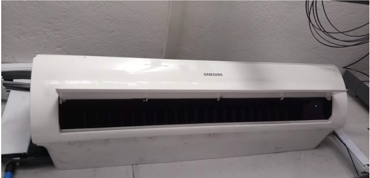
Figure 8: A split air conditioner
