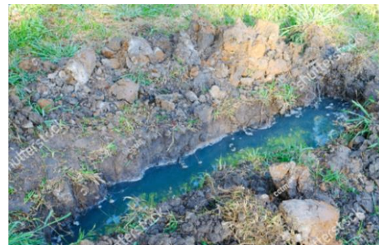
Figure 21: Physical damage of the system with the first-hand release of raw sewage
