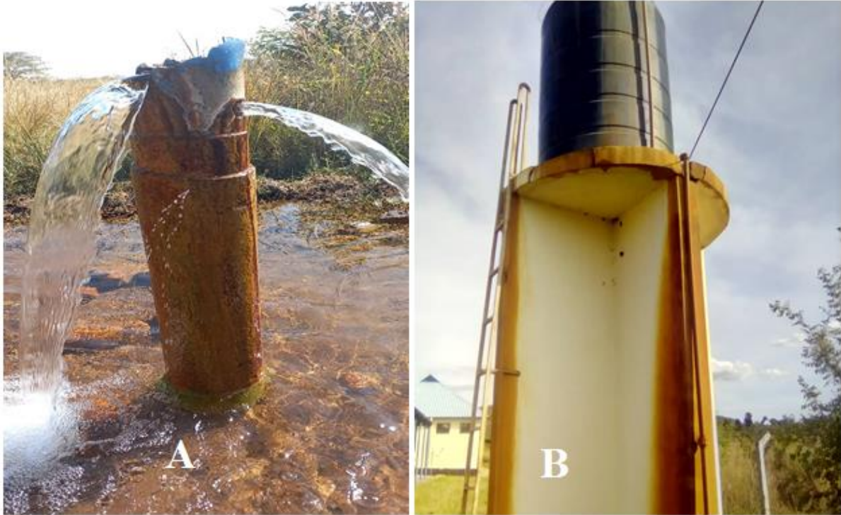
Plate 1: (A) A borehole that has been abandoned because of water metallic taste and (B) an example of a typical discolouration caused by Fe-contaminated groundwater to the concrete tank raiser found in the study area (Source: Mkelemi field survey, 2022)
