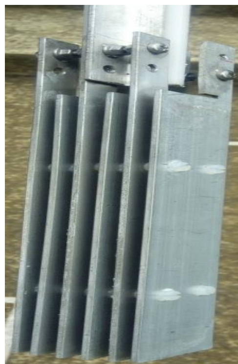
Figure 7: Power supply in a parallel monopolar connection
